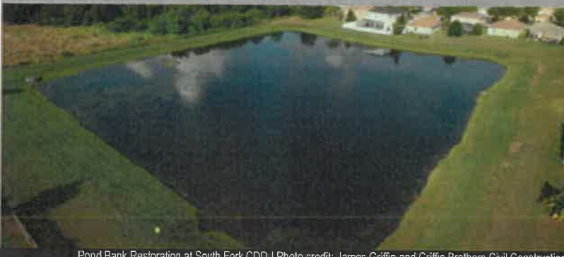
Pond Bank Restoration at South Fork CDD | Photo credit: James Griffin and Griffin Brothers Civil Construction
