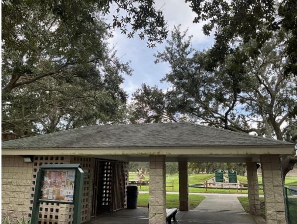
Asphalt shingle overview with discoloration at shingles and fascia board
