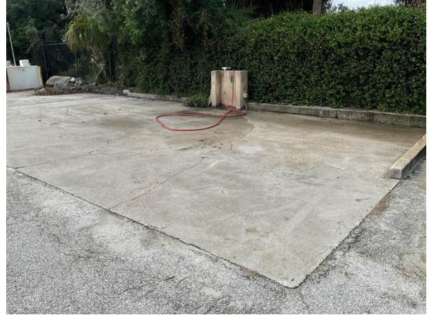
Concrete cracks at wash station
