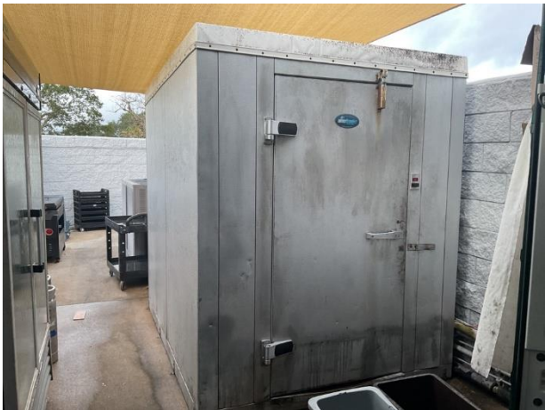
Existing walk-in freezer
