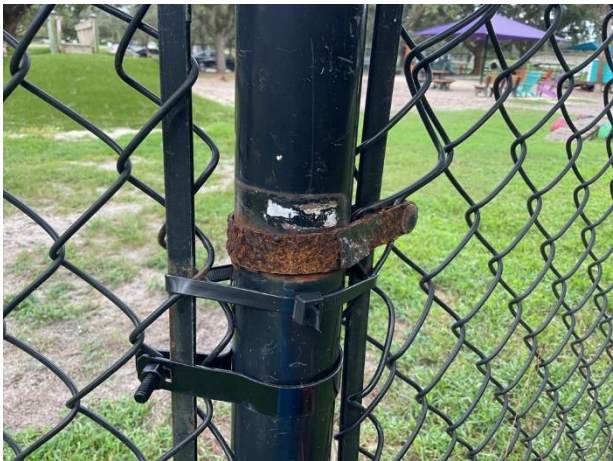
Rust at fence hardware
