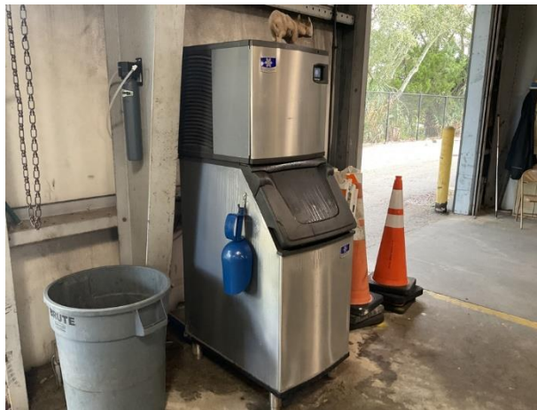
Ice machine at maintenance building
