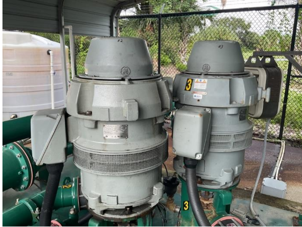
General electric irrigation system pumps
