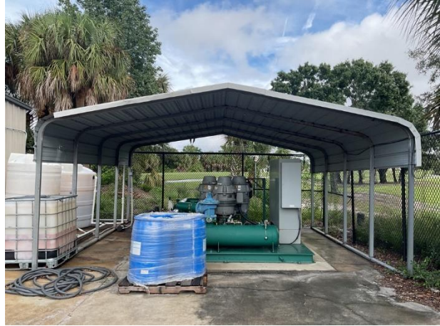
Irrigation system pump station
