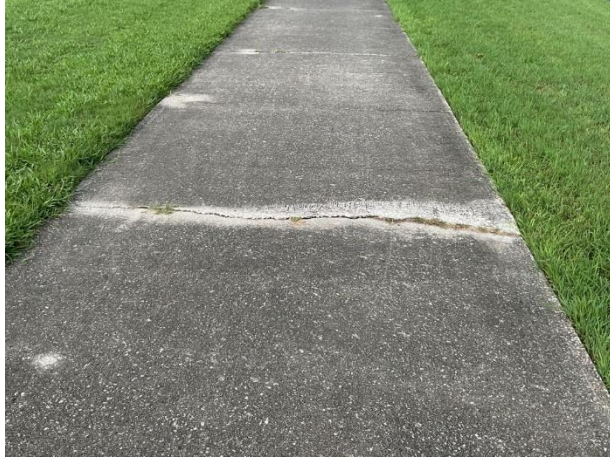
Evidence of previous repair at Woodside Park
