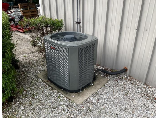
Split system condensing unit at maintenance building
