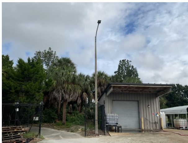
Light pole with LED fixture
