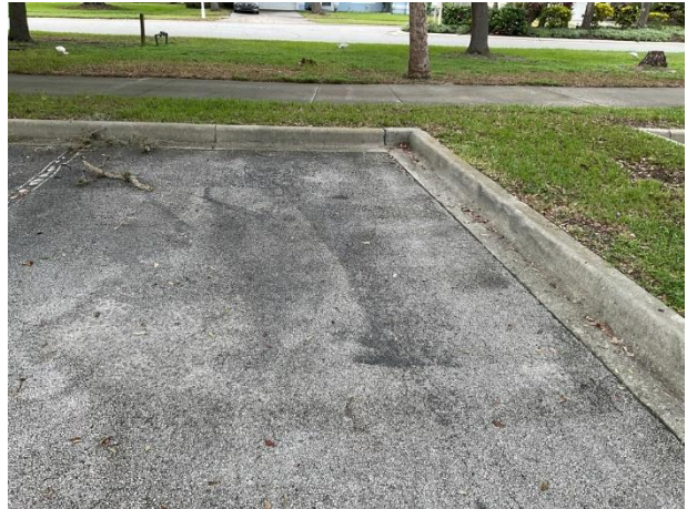
Evidence of historical seal coat application
