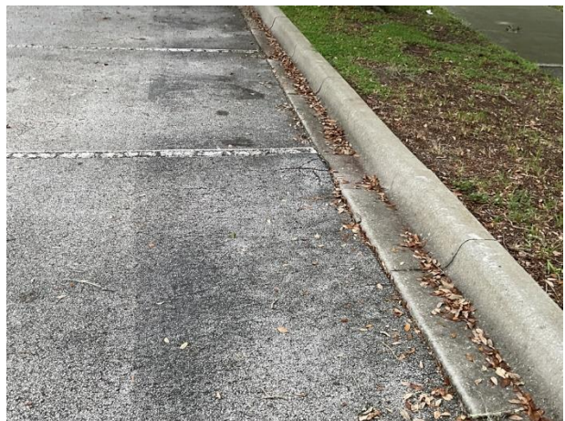
Evidence of tree root intrusion
