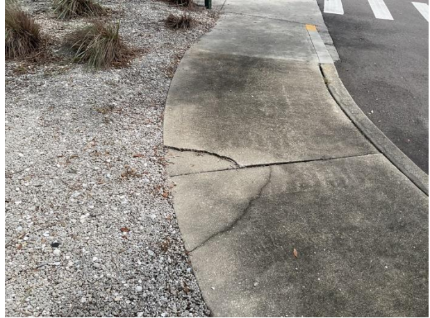
Sidewalk trip hazard
