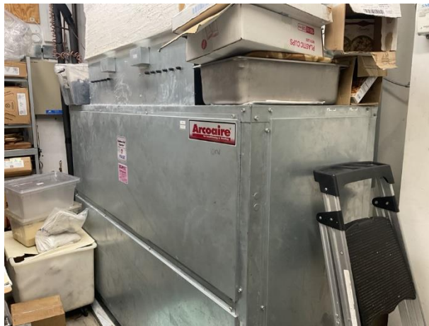
Air handling unit at restaurant
