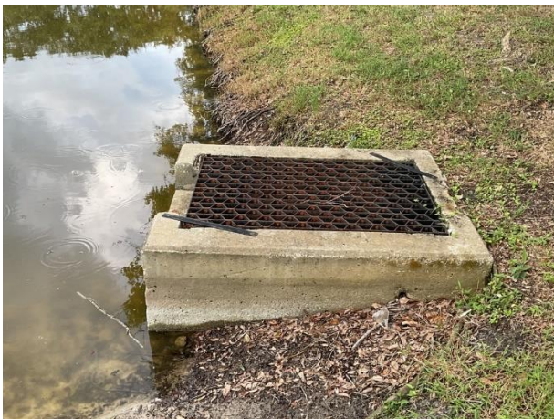
Pond control structure near Woodside park
