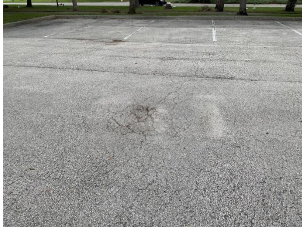
Pavement cracks and settlement
