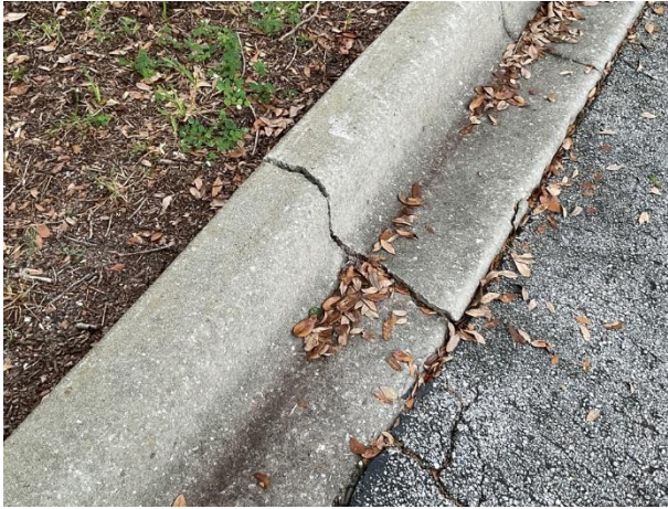
Concrete crack with tree root upheaval at Woodside Park
