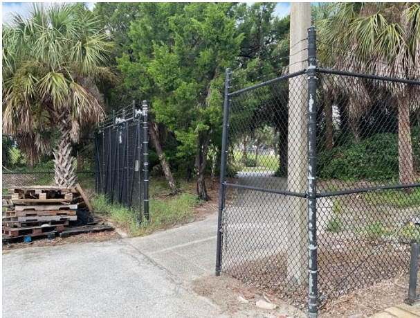
Rear gate at maintenance facility with finish deterioration
