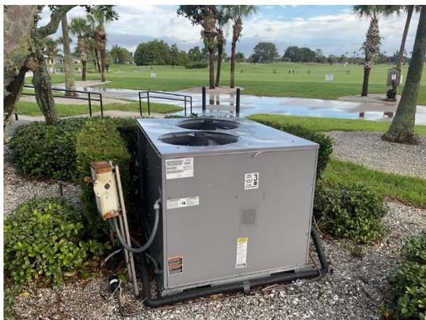
Condensing unit at pro shop and offices
