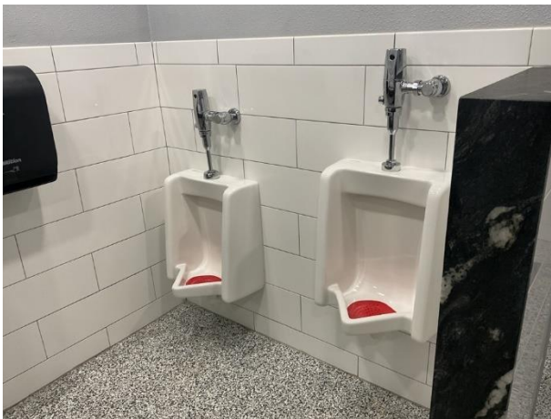
Rest room fixtures
