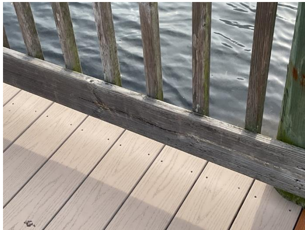
Wood deterioration at stringer
