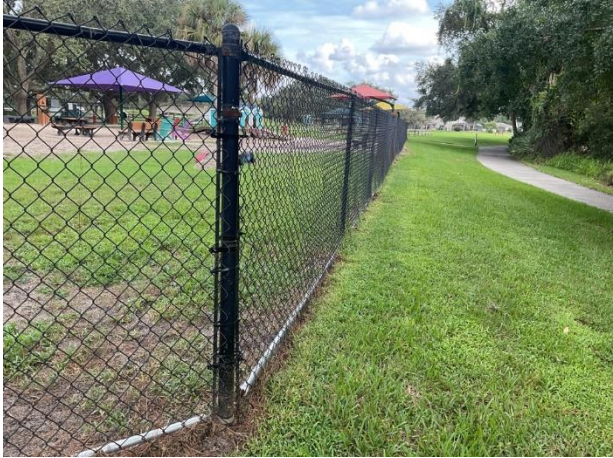
Chain link fence at dog park with warped webbing
