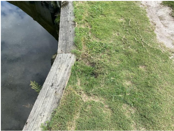
Erosion at backside of Hole 7 bulkhead
