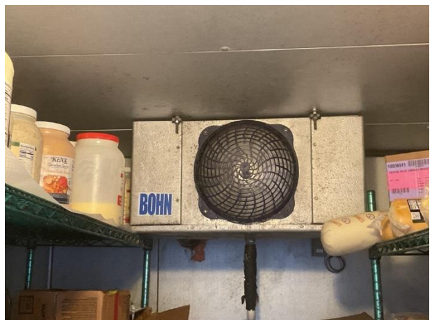
Freezer mechanical equipment
