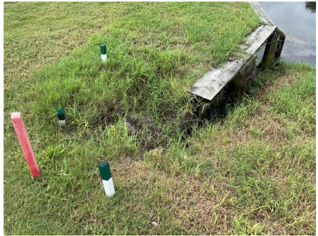
Erosion at end of Hole 7 bulkhead
