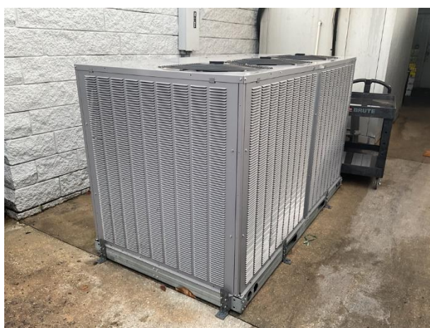
Condensing unit at restaurant
