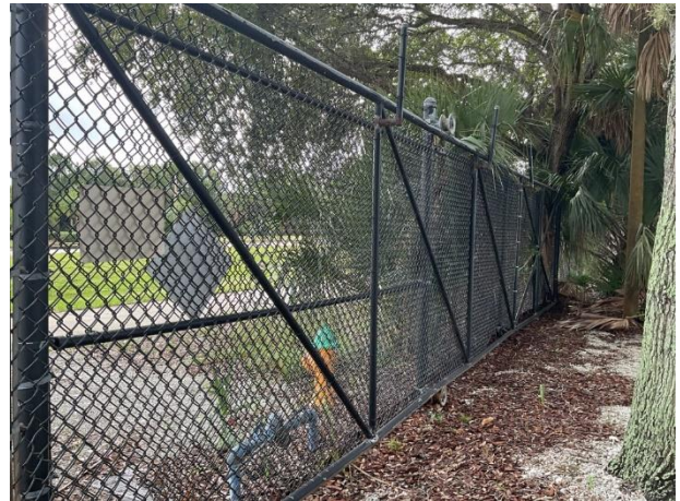
Rolling gate at maintenance facility
