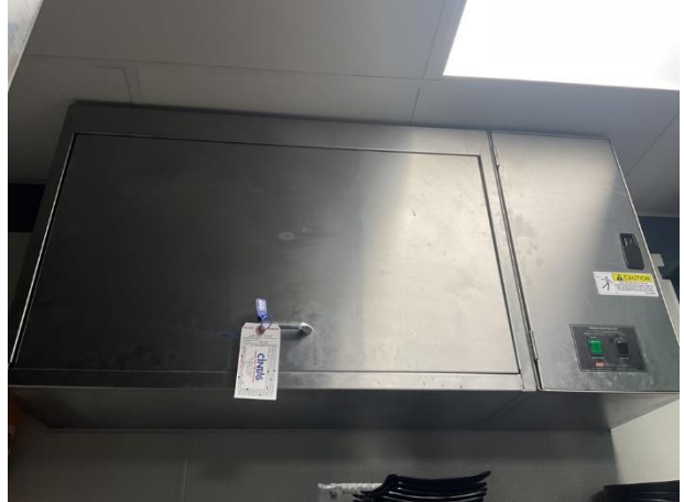
Range hood control system
