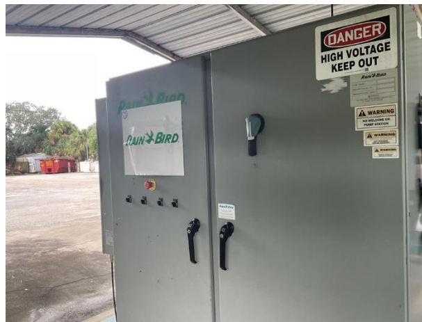
Pump control system
