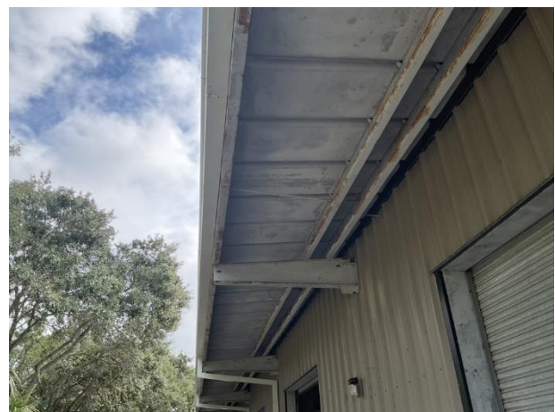
Structural steel frame with rust evident
