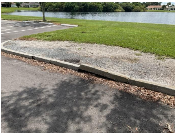
Concrete curb upheaval at the Clubhouse parking area
