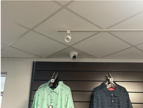
Security system camera
