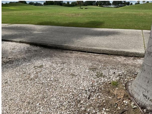
Soil undermining cart path at graveled area
