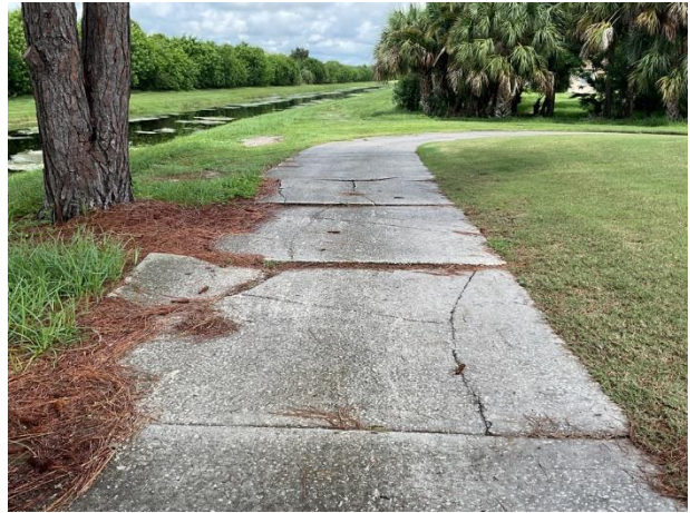
Significant tree root intrusion near hole 11 tee area
