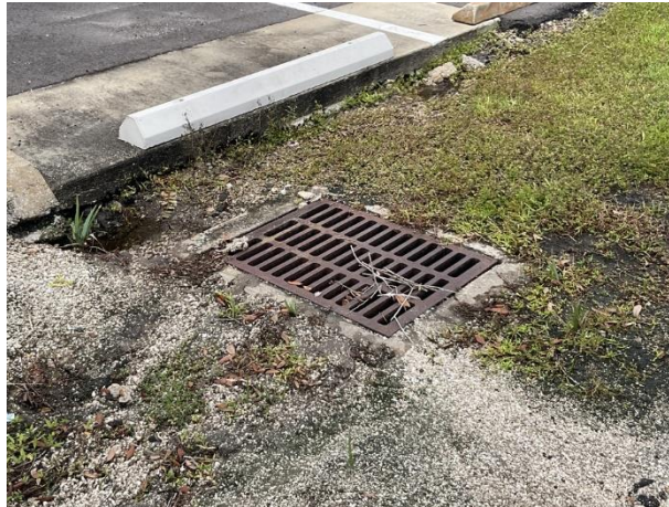
Landscape catch basin at clubhouse parking area
