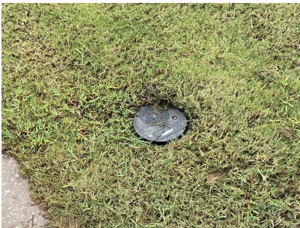
Irrigation system control valve
