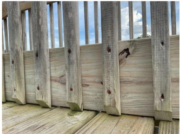
Rust at visible screwheads at railings
