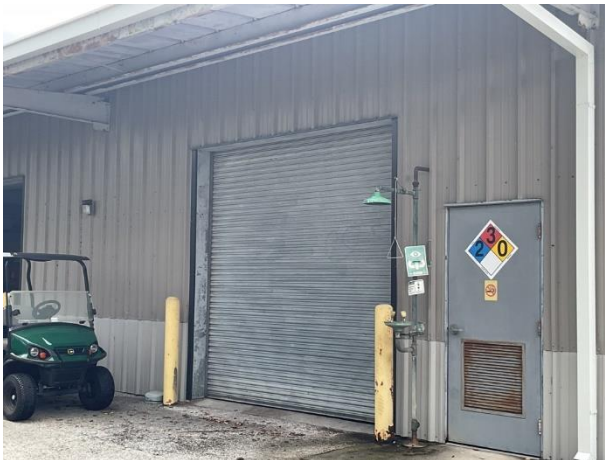
Rolling door at attached fertilizer storage room
