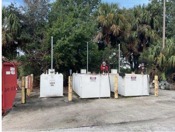
Gasoline, diesel fuel and oil separation storage tanks
