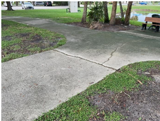
Concrete cracks and trip hazards near playground
