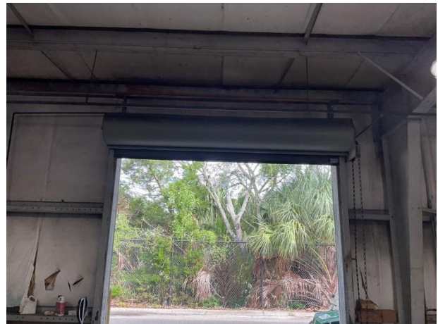
Rolling door at maintenance shop
