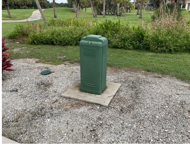
Irrigation system controller near Hole 6
