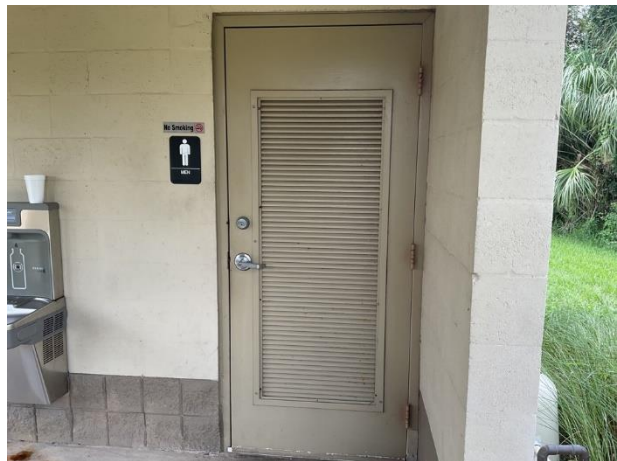
Rest room door with rust evident
