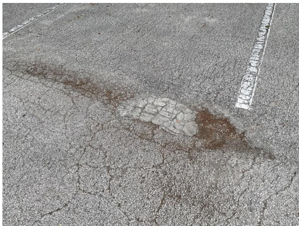
Evidence of previous attempted repair
