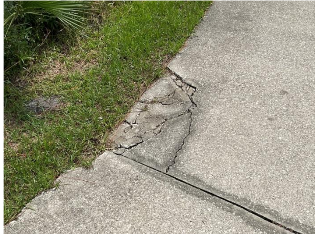
Concrete walking trail settlement
