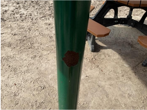
Rust at frame
