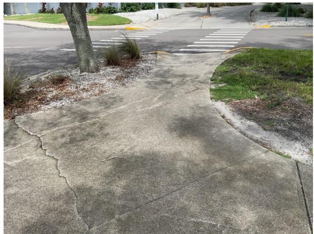
Concrete sidewalk with cracks and trip hazards at Clubhouse
