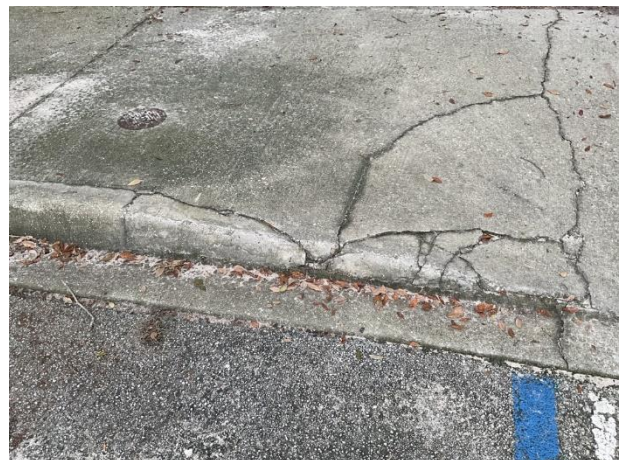
Concrete deterioration at Woodside Park
