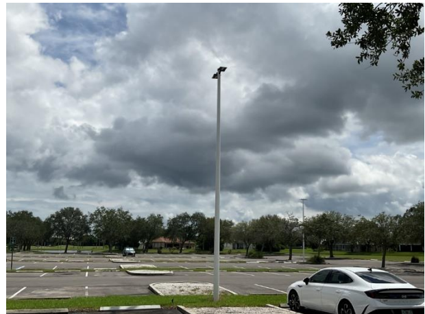
Light pole with LED fixtures at the clubhouse parking area
