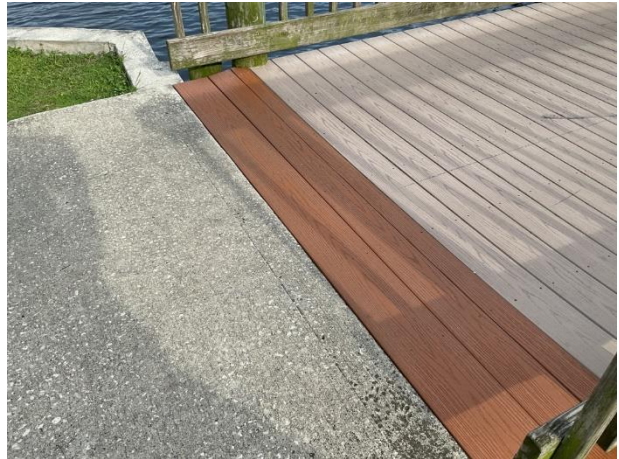
Evidence of previous partial replacement
