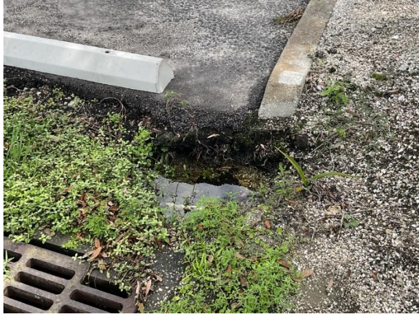
Soil undermining pavement at drainage area
