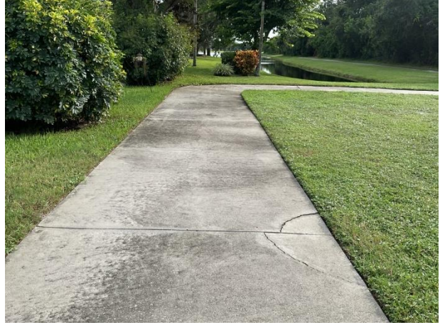
Concrete sidewalk with cracks and settlement near Fawn Ridge
