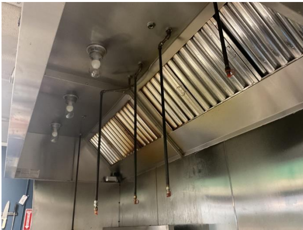
Range hood with integrated fire suppression system
