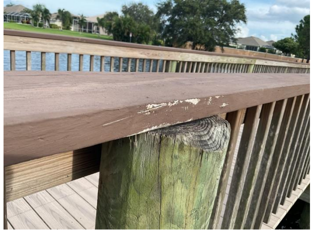
Railing finish deterioration
