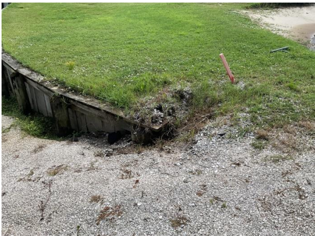
Erosion at end of Hole 7 bulkhead
