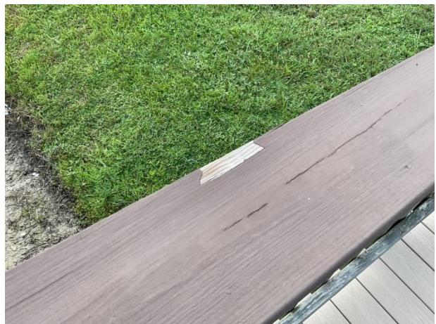
Handrail coating deterioration
