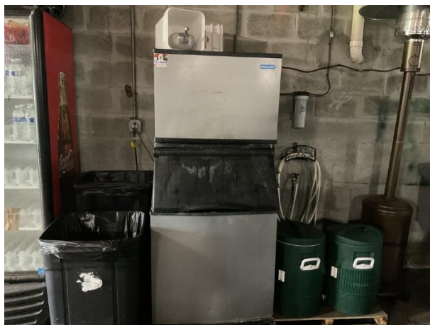
Ice machine at cart barn
