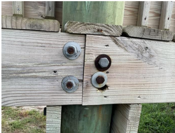
Rust at fasteners
